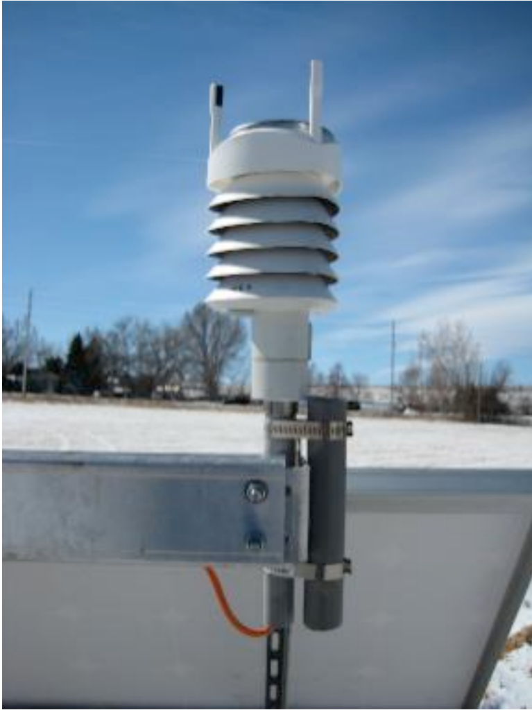
Example 3 - Vaisala mounting pipe is hoseclamped to an adjacent section of PVC, against a solar panel mount.
