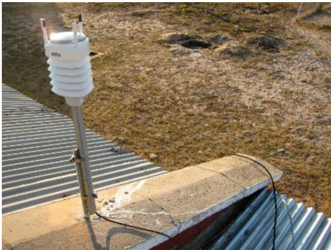
Example 1 - Vaisala hose clamped to \frac{5}{8} inch rod grouted into roof.
