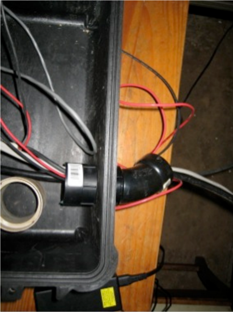
Plastic two" pass-through for cables routed from the GPS antenna, Vaisala weather station, solar panel, and battery
