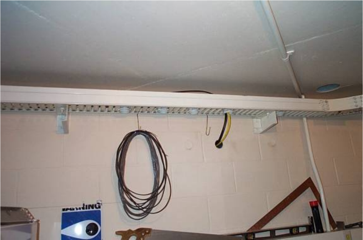
Area where the MET and antenna cables enter the observatory.
