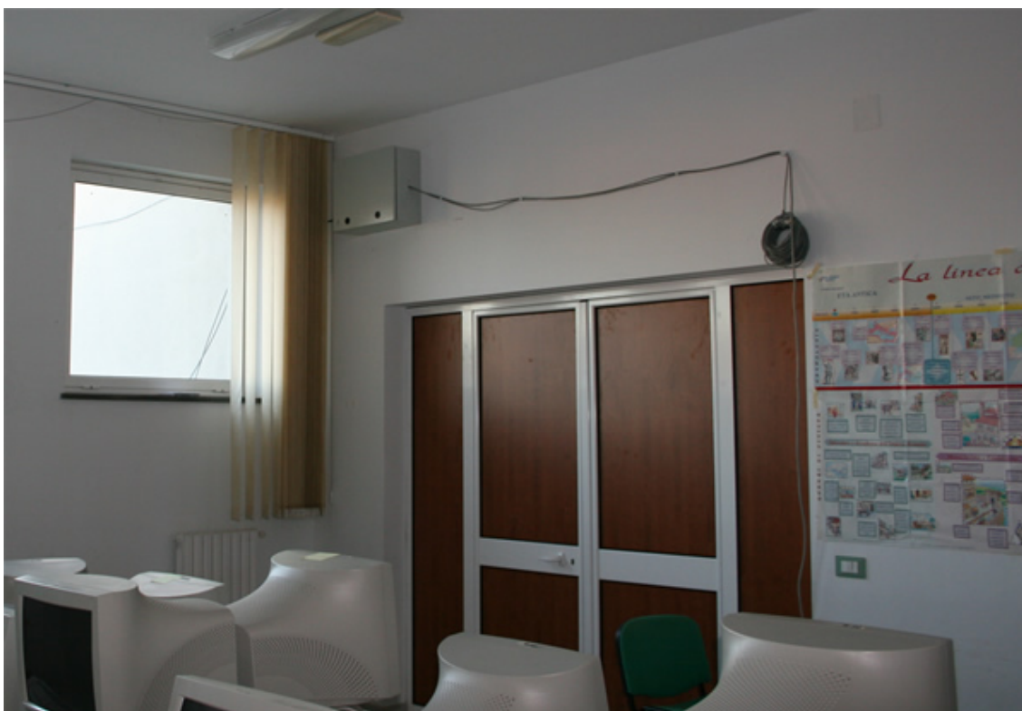
Wall mounted enclosure used in Calabria, Italy (site TVRN).
