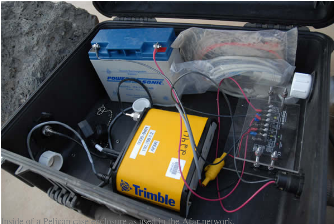
Inside of a Pelican case enclosure as used in the Afar network.
