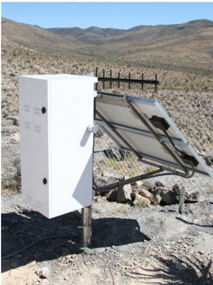
SunWize enclosure as used in the Plate Boundary Observatory and in the BARGEN network.
