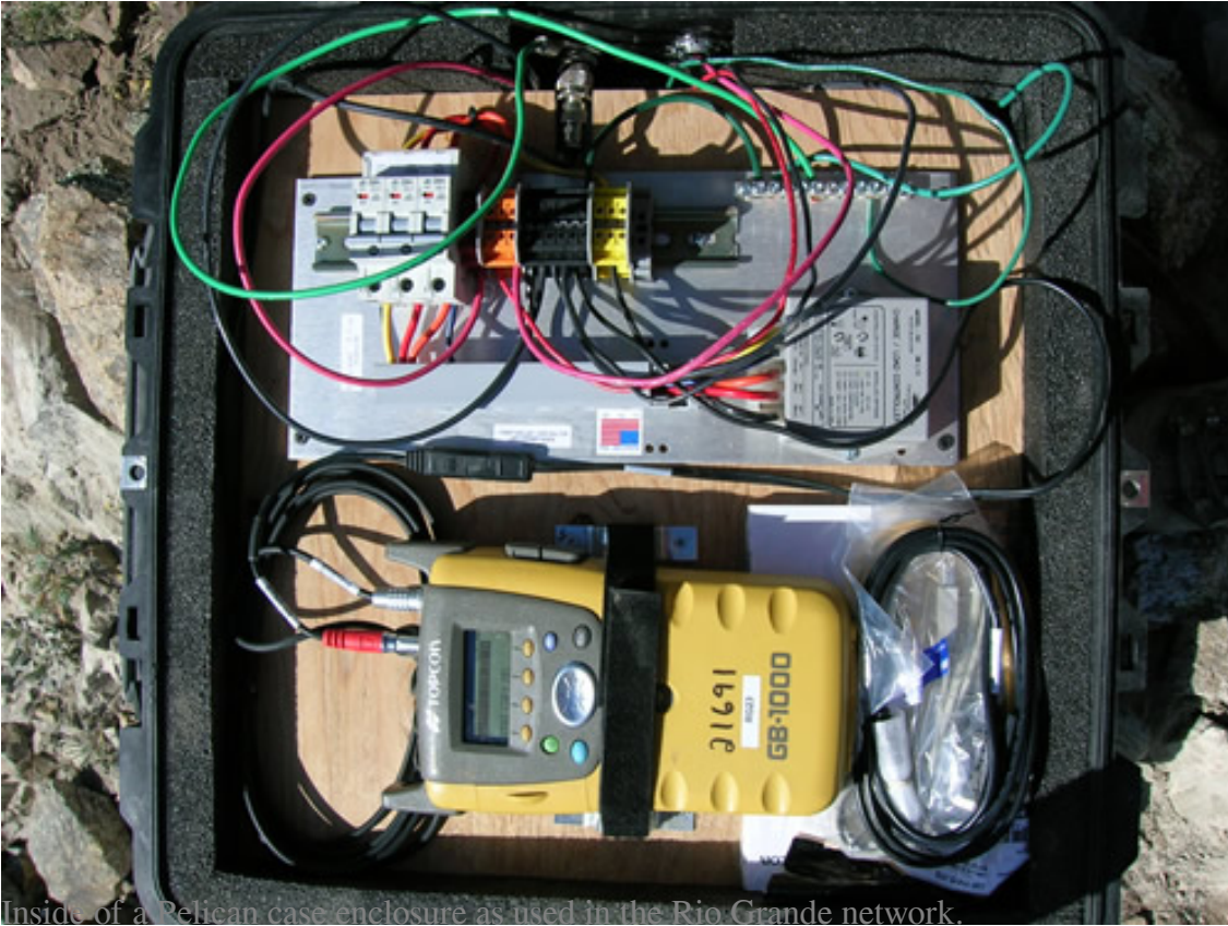
Inside of a Pelican case enclosure as used in the Rio Grande network.
